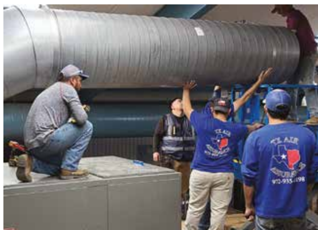
Corey Robinson, of TX Air Assurance, Inc., and his team donate their labor installing new equipment at Bridges Training Foundation.
